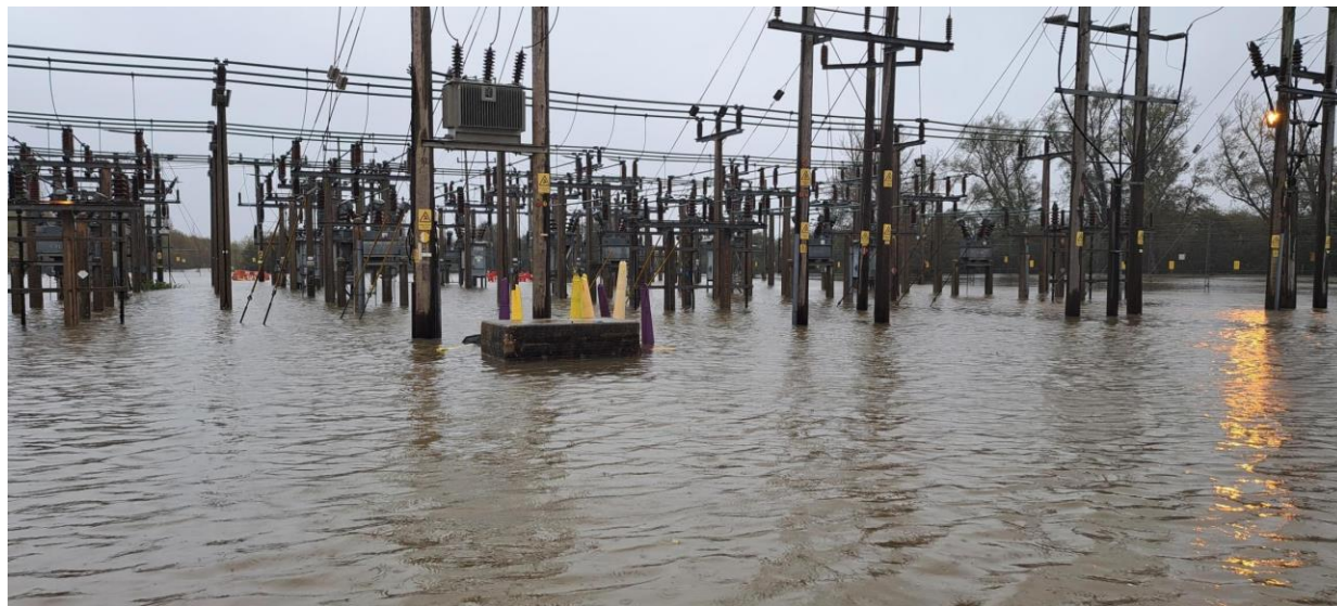
Figure 1: Flooded yard at Bognor Regis
